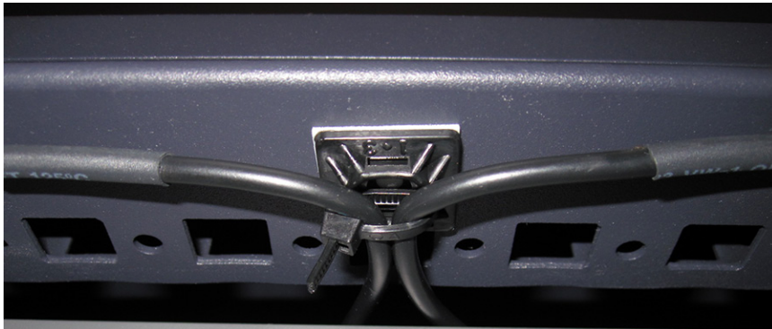
Figure 15: Tie-Wrapped Connector Wires
